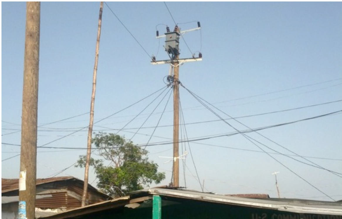
Figure 5: Example of MV Distribution Approach of LEC using dedicated drop down lines.
